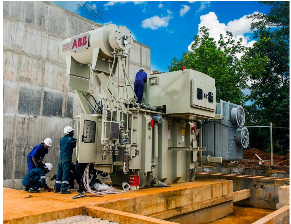
New Namugongo substation completed in 2015 (US$6m)
